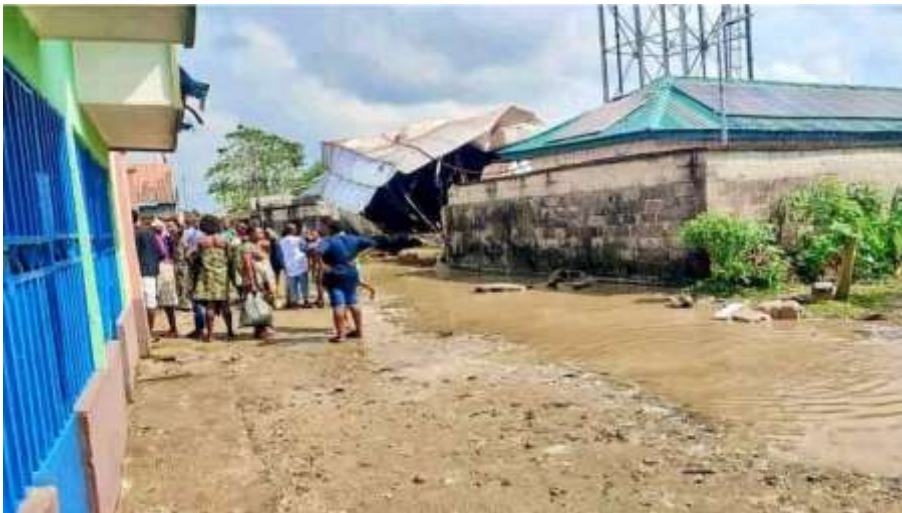
Plate 2.9: The recent collapse of a water tank built by the Hydrocarbon Pollution Remediation Project (HYPREP) in the Gwara area of Ogoni in Rivers State
