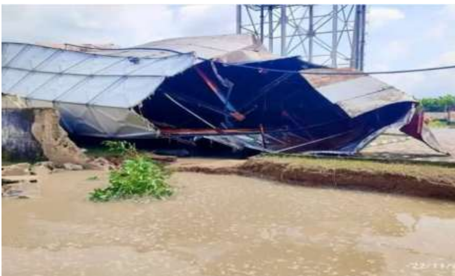
Plate 2.10: The recent collapse of a water tank built by the Hydrocarbon Pollution Remediation Project (HYPREP) in Eleme area of Ogoni in Rivers State.
