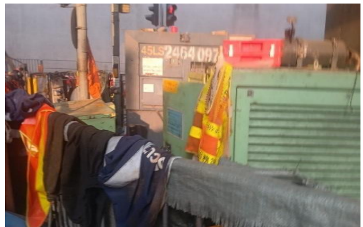
Figure 2: Emergency diesel generator
