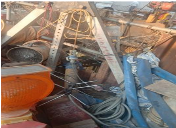
Figure 1: Blow fan and flexible air duct
