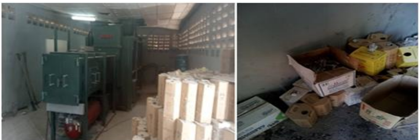
Figure 1 – Incineration plant, Gombe
