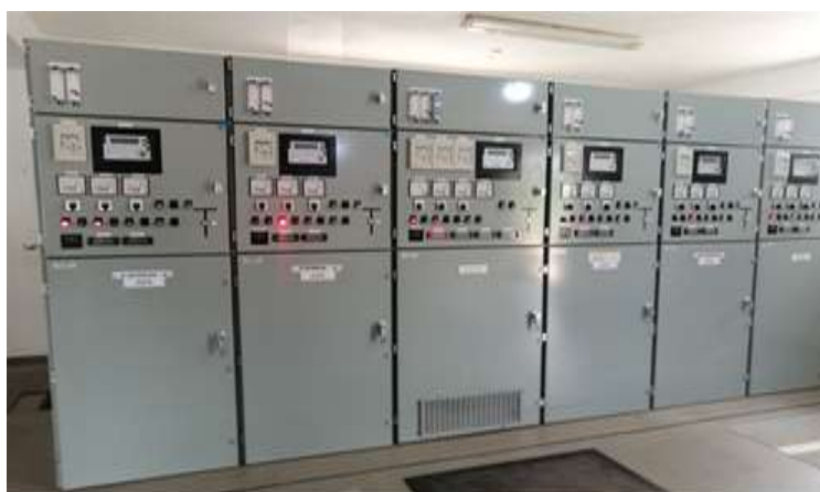
Fig. 3 Atoabo Substation 11 kV Indoor Panels
