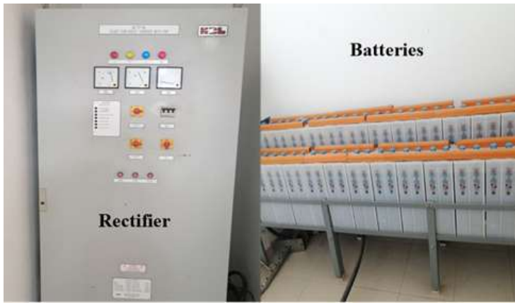
Fig. 4 Atoabo Substation Rectifier and Batteries
