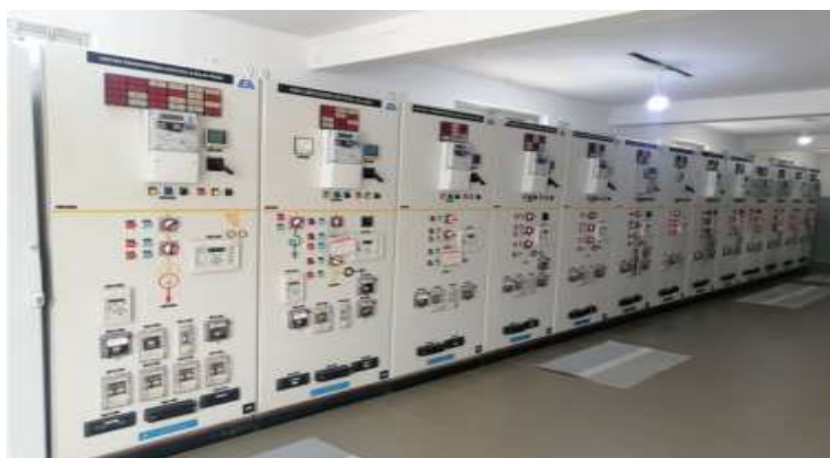
Fig. 2 Atoabo Substation 33 kV Indoor Panels
